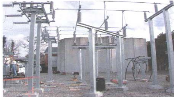
Portion of new 69 kV Bus Tie at the Logan Substation in Shrewsbury.
